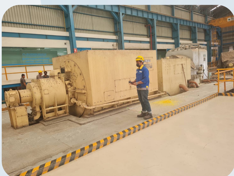
Major Overhaul Synchronous Generator 25 MW
