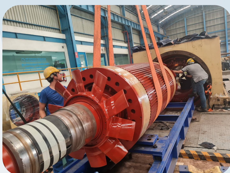
Major Overhaul Synchronous Generator 25 MW
